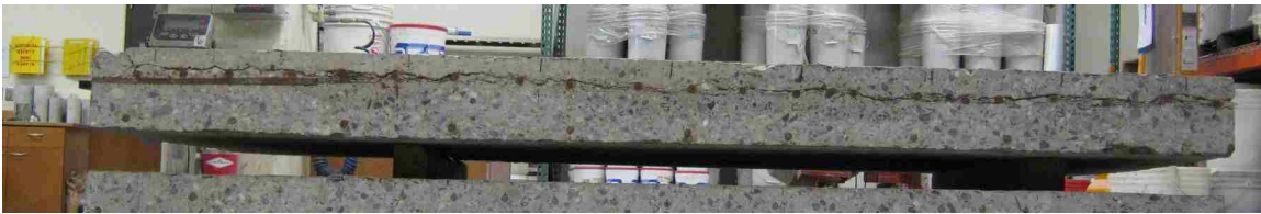
Figure 2-3: Delaminated concrete bridge deck slab.
